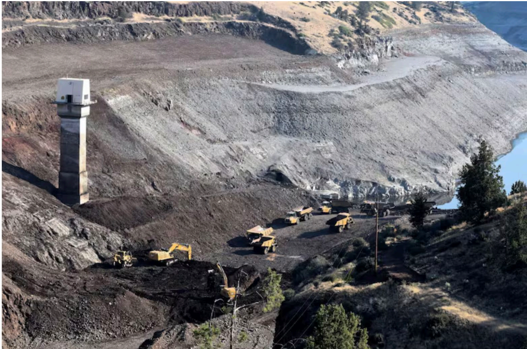
Scoop by scoop, crews from construction company Kiewit are deconstructing the massive earthen barrier that was Iron Gate dam, July 26, 2024.
