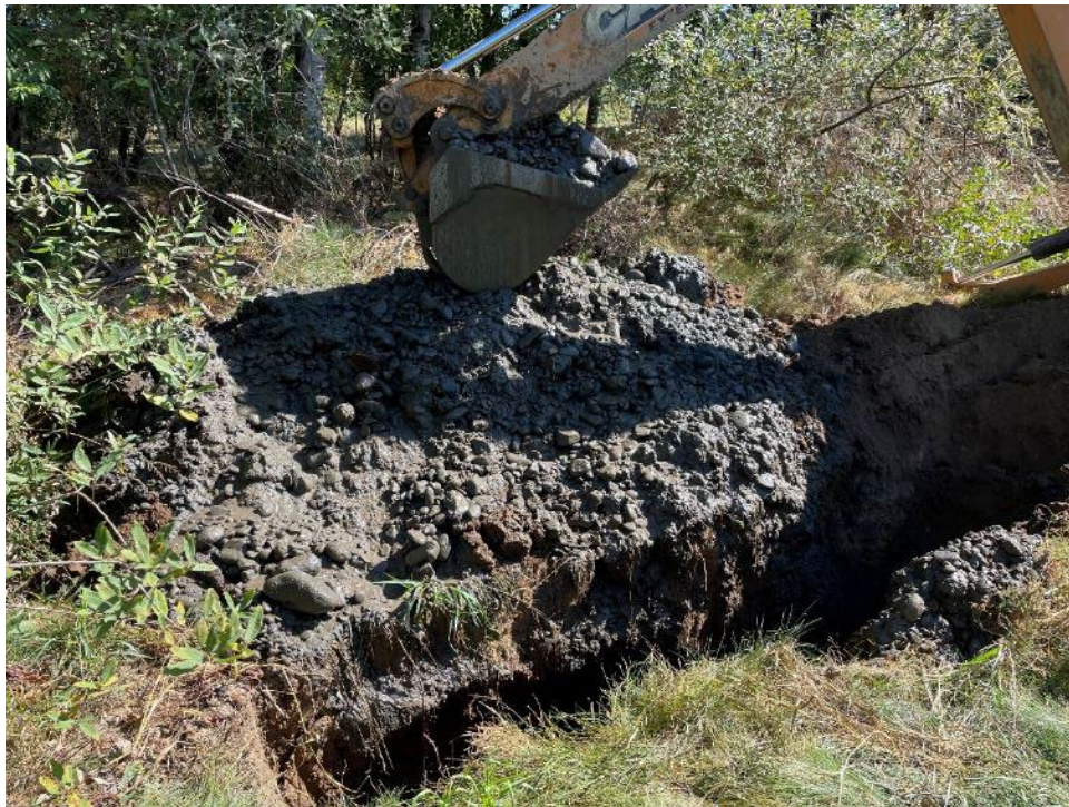
Top - coarse alluvial layer below 5 feet depth. Bottom – spoils pile showing primarily the coarse alluvial sandy gravel layer below 5 feet depth.
