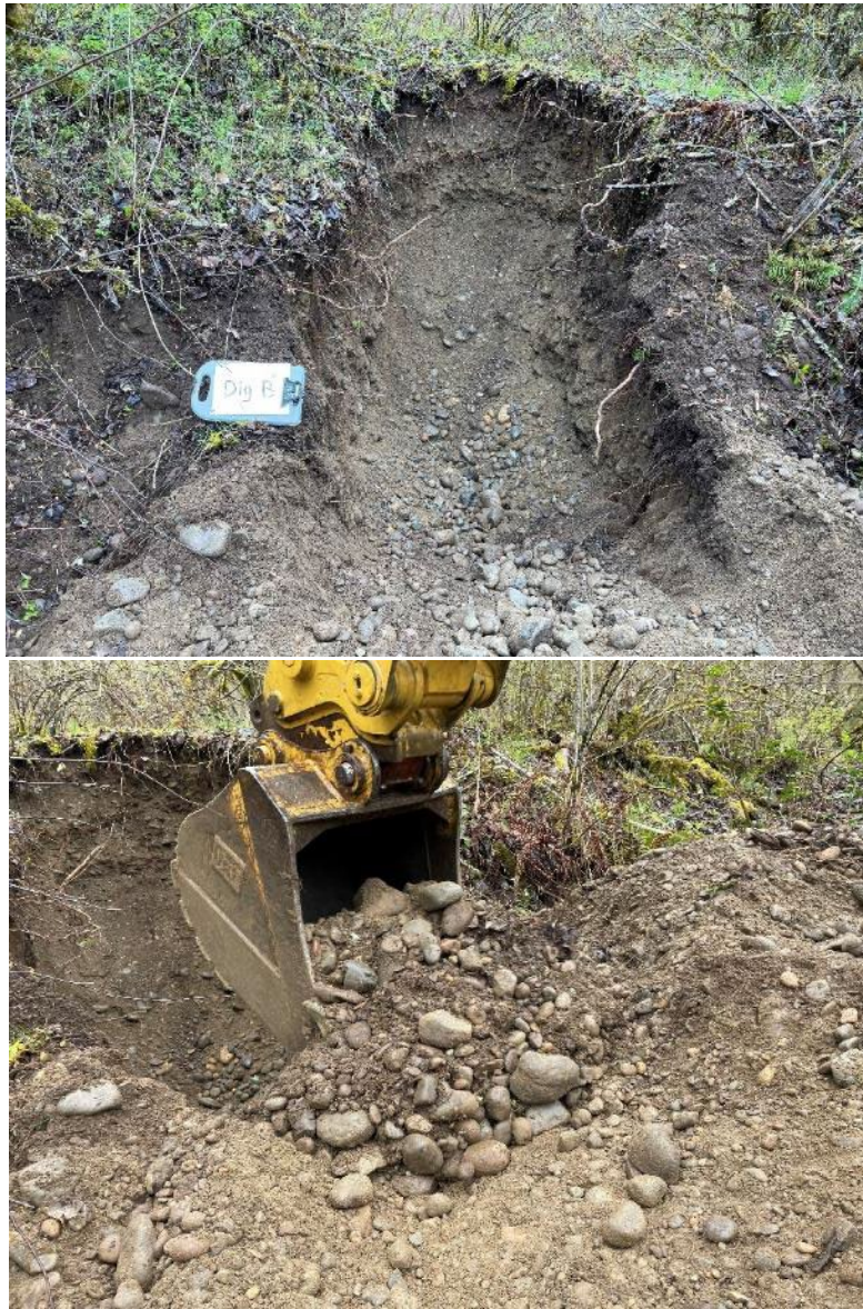
Top – Gravel mixing into loose fines.
