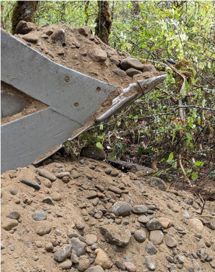
Top - Sandy loam with thick roots at top of pit; Bottom - close up of cobbles at 3 feet
