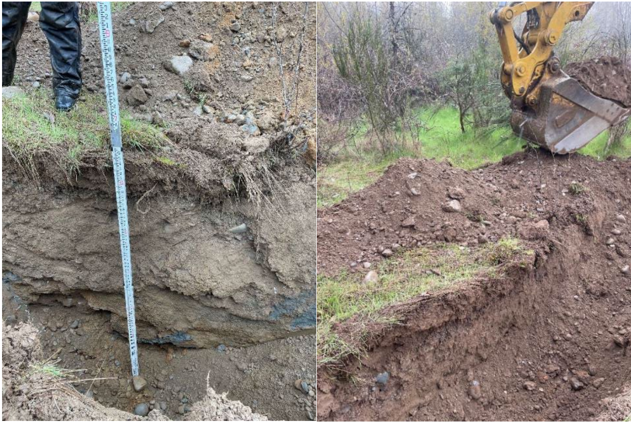
Left - Silty sand above gravel and cobbles layer. Note gray clay mixed into sand layer.
